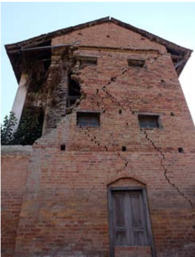
Absence of ring beams causing the cracks at the Bhaktapur Durbar Square
